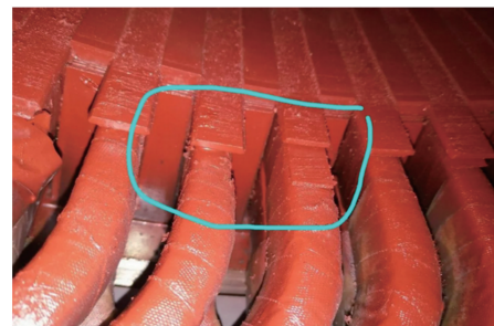
Fig.1 Wear of stator slot wedge
